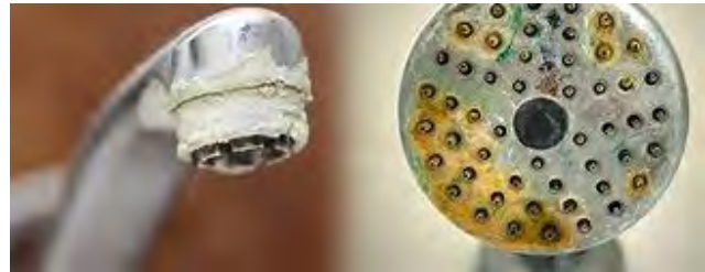
Buildup of limescale on fixtures
